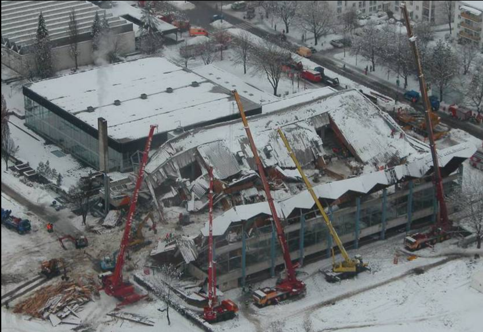
Eishalle Bad Reichenhall – Progressive collapse under char. snow load
